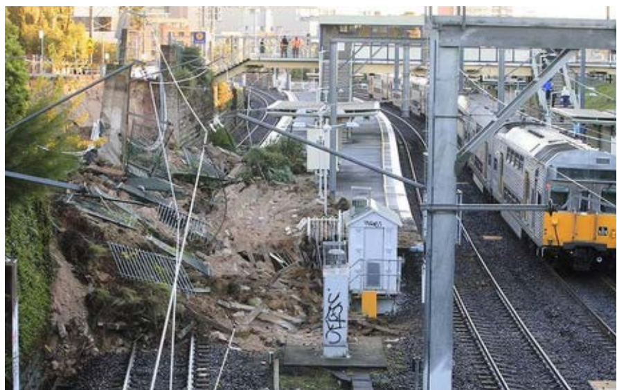
Nine days of extreme rainfall in 2013 caused a retaining wall to collapse at Harris Park train station. Photo: Carlos Furtado
