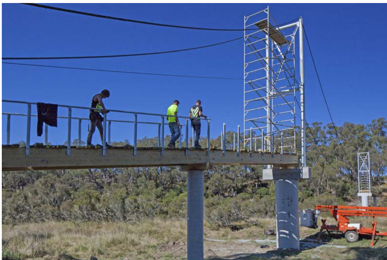
Apsley Falls bridge construction, Oxley Wild Rivers National Park. Photo: Gerhard Koertner/DPIE
